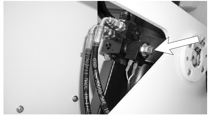
Figure 7.21.1 - Emergency Lower Valve, Controlling Lower Boom
