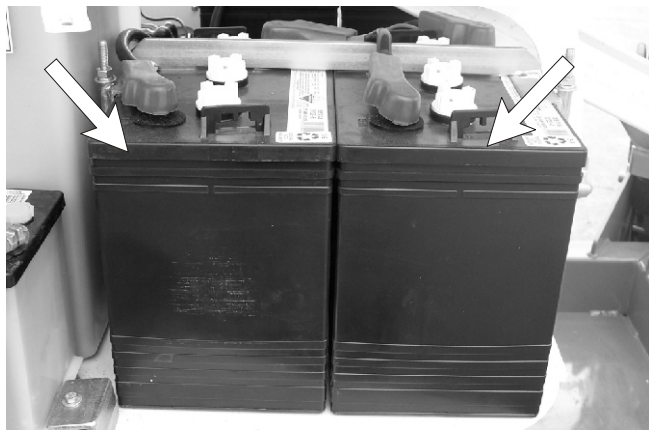
Figure 11.6 - Two DC Motor Batteries (Petrol/Diesel Engine Side)
