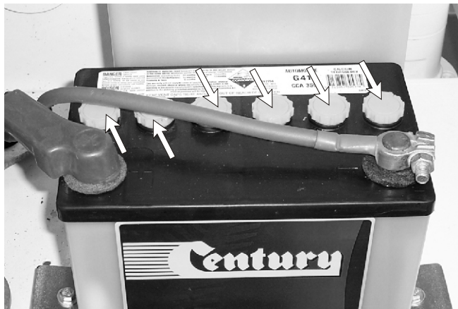
Figure 7.7 - Battery Fluid Level
